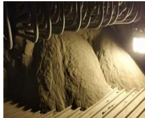
Ash Deposition at Low Loads
